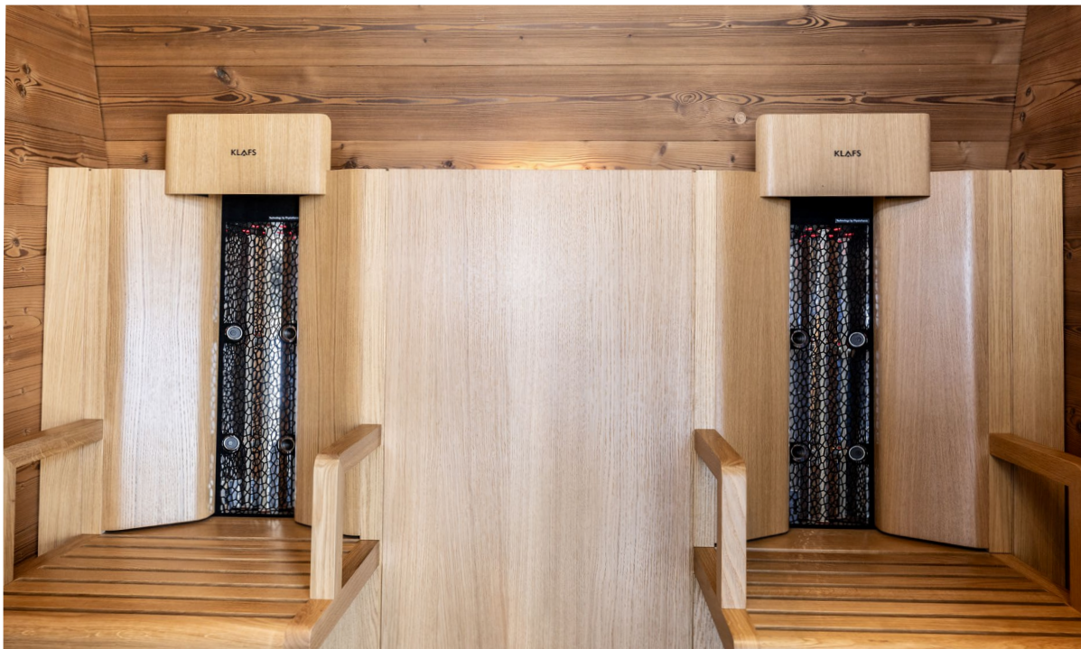
Flexibel installierbare InfraPLUS SMART SEATs | © Nikolai Milatovic Photography, Merkur Gym
